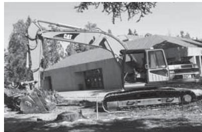
KRESGE AUDITORIUM CAME DOWN TO MAKE WAY FOR THE NEUKOM ACADEMIC BUILDING AT STANFORD LAW
